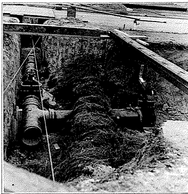
16" CITY WATER DISTRIBUTION
