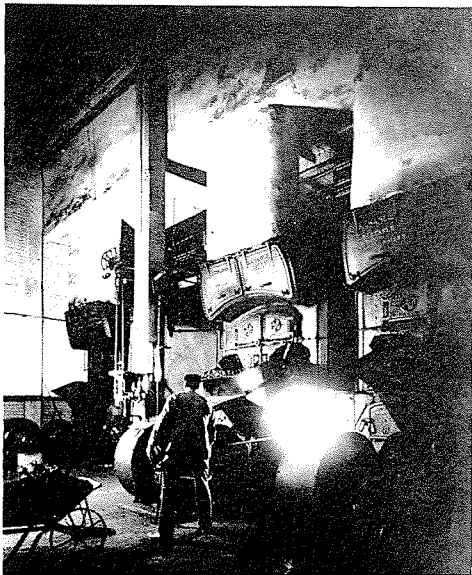
The Boiler Room
